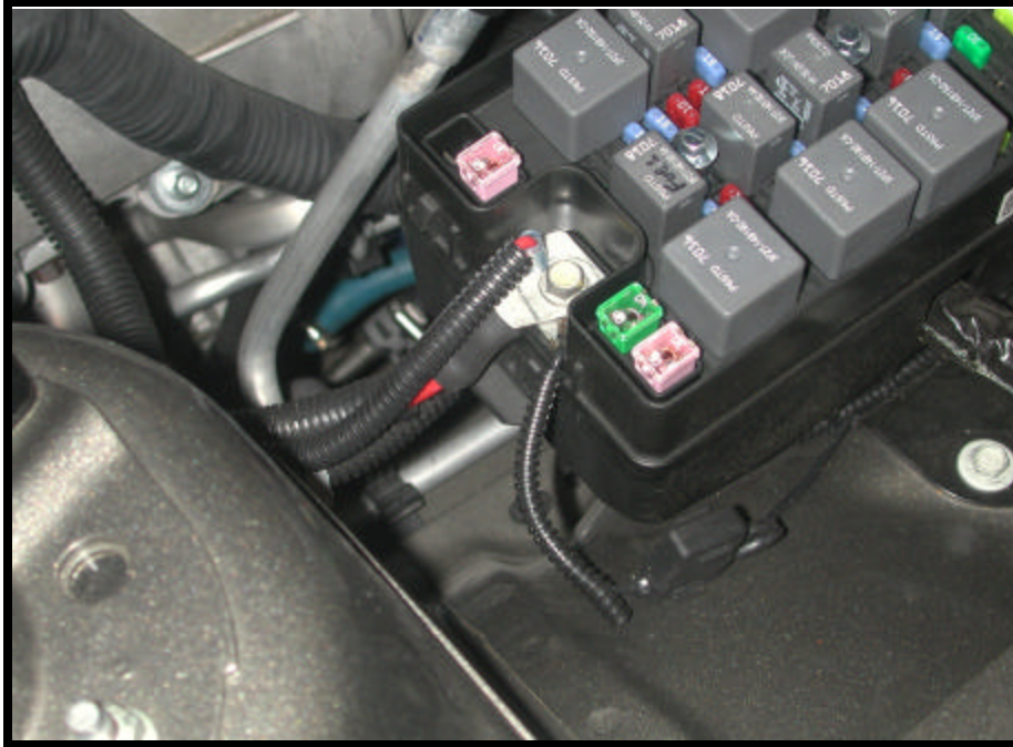
Photo 6: 12V Power Supply Connection
