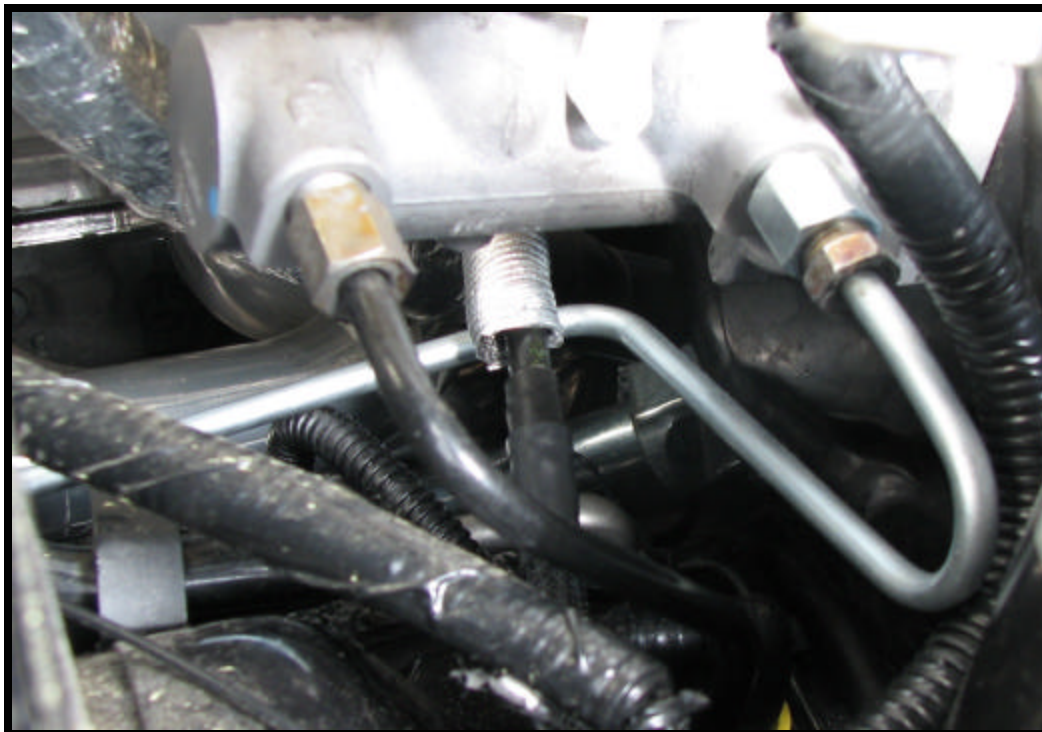
Photo 4: Master to Solenoid Line Routing Path- Master View
